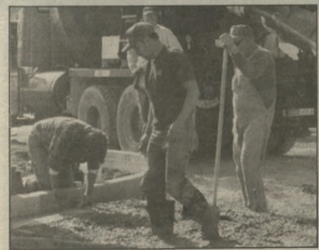
Workers, left, build the drive up ramp for the ATM station. A worker, right, measures the wooden frame at the ATM site.
